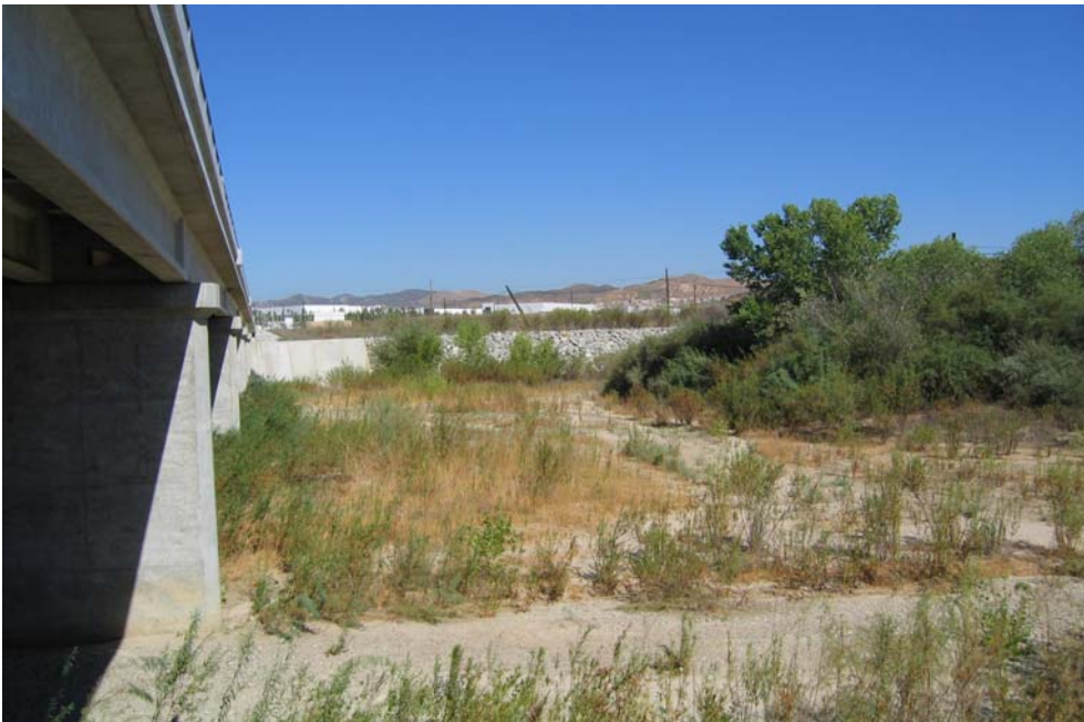
Photo 2. Upstream of Commerce Ctr. Drive Bridge looking North at the concrete/riprap bank protection for Hasley Creek
