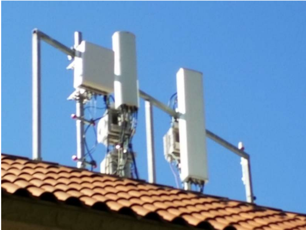
Antennas on building Beta Sector
