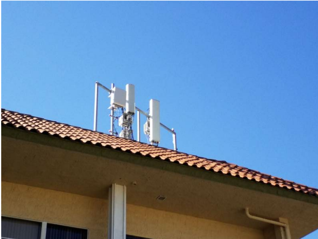
Antennas on Alpha Sector
