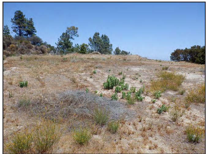
Photo 4 – The graded pad is shown. The undocumented fill to be removed is visible on the pad in the background. View faces northeast.
