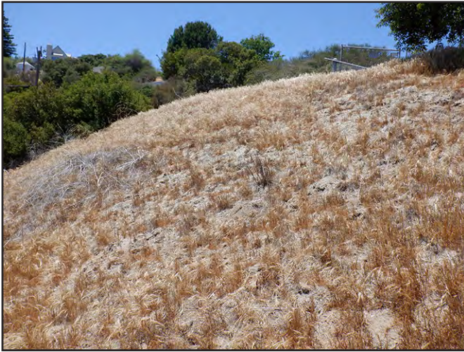
Photo 1 – The undocumented fill at the entrance slope is shown. View faces west.
