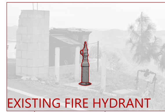
EXISTING FIRE HYDRANT
