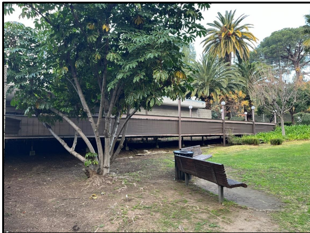
East elevation bridge, facing west. Bridge expected to remain, materials replaced in-kind if necessary.
