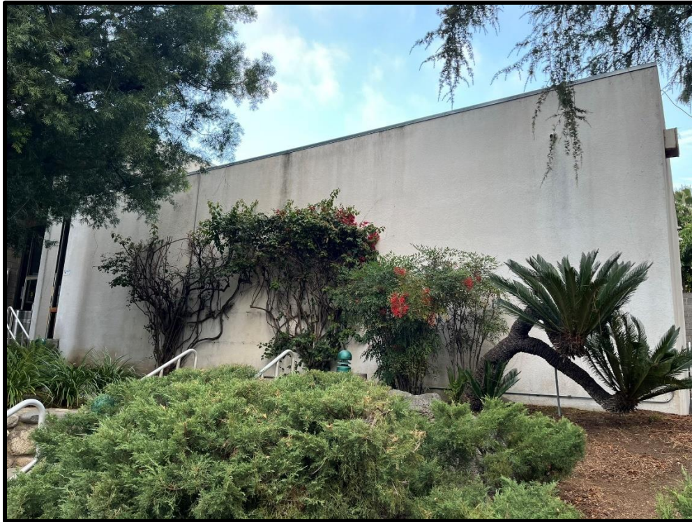
South elevation of community room, facing north. New deck will be located on this elevation, with a shade canopy and sliding doors. New fenestration will be added to east and north elevations of the community room.
