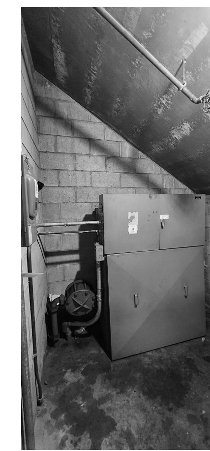
1 ELEVATOR CONTROL ROOM EQUIP.
