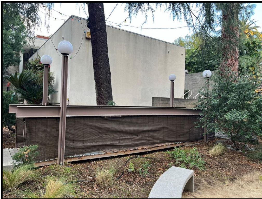
South elevation bridge and east elevation of community room, facing northwest. Bridge expected to remain, materials replaced in-kind if necessary. New fenestration is proposed on east elevation of community room.
