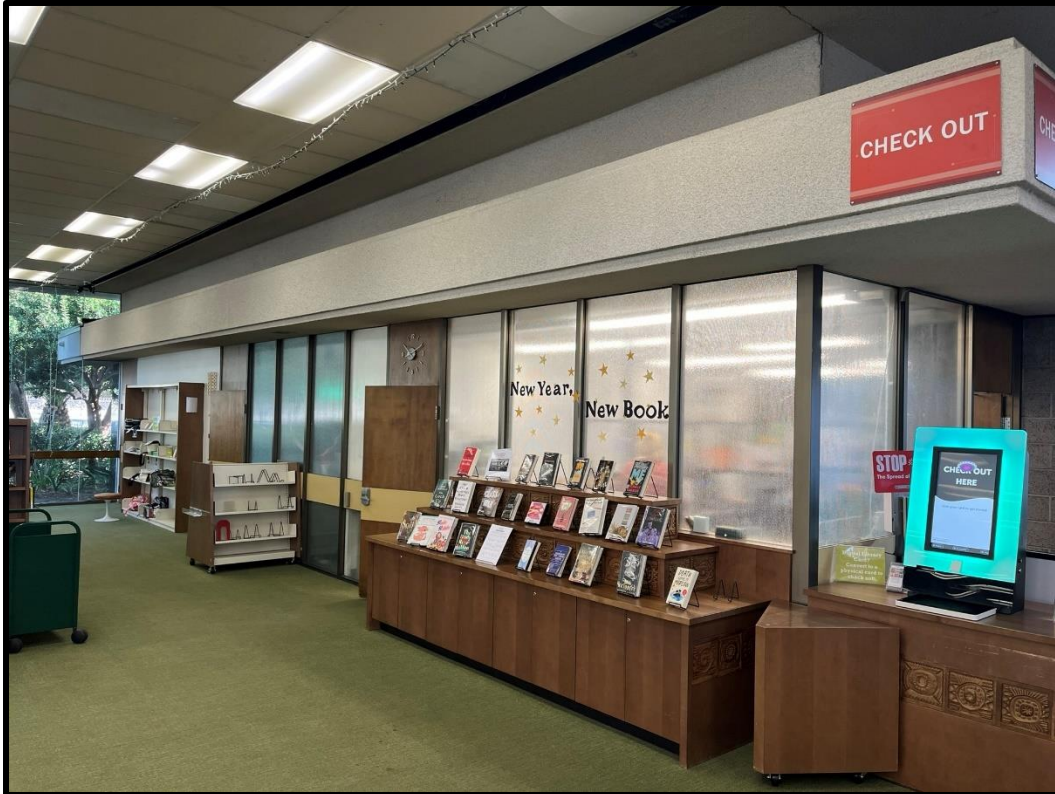
Office on eastern portion of main floor, facing northeast. Walls, doors, and existing windows will be removed and replaced. Space will be reconfigured.
