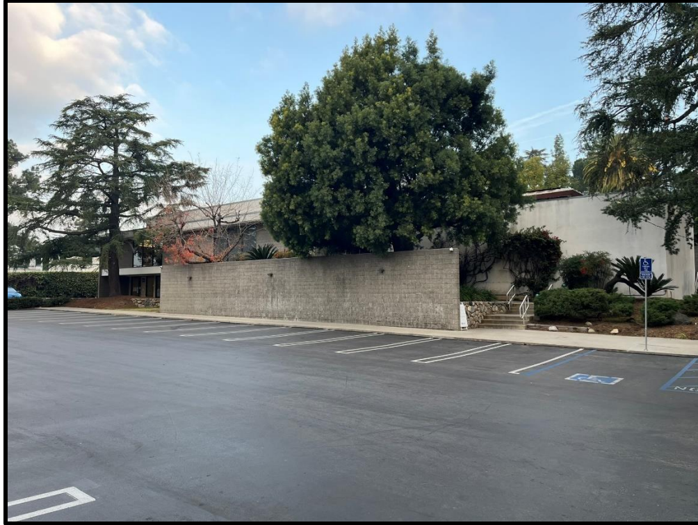
South elevation, facing northwest. New two-story atrium/entrance and deck will be located on this elevation.
