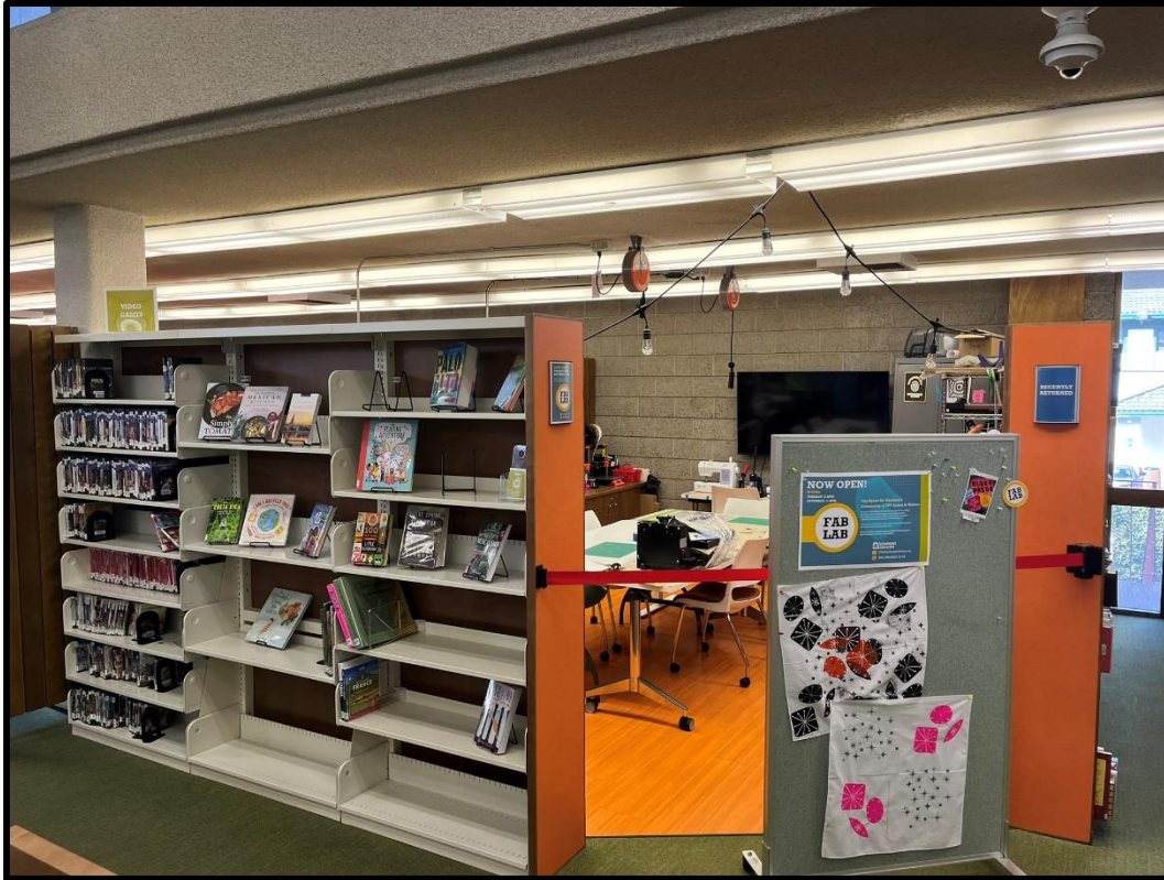
Office on western portion of main floor, facing northeast. Walls, doors, and existing windows will be removed and replaced. Space will be reconfigured.
