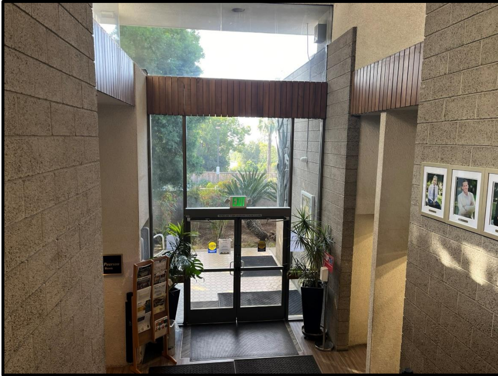
Interior view of south elevation entrance. Community room access on the left of image, bathrooms on the right of image. Space will be significantly modified.
