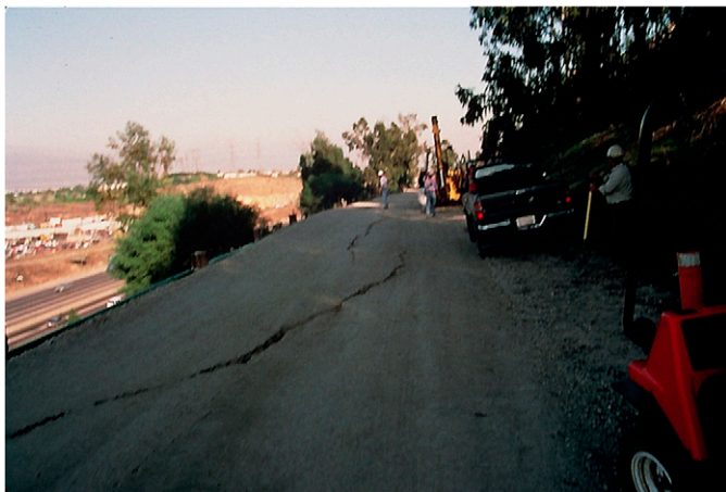
Fig. 2. Cracking on a north slope bench following the 1994 Northridge earthquake (Photograph courtesy of Raymond B. Seed)
