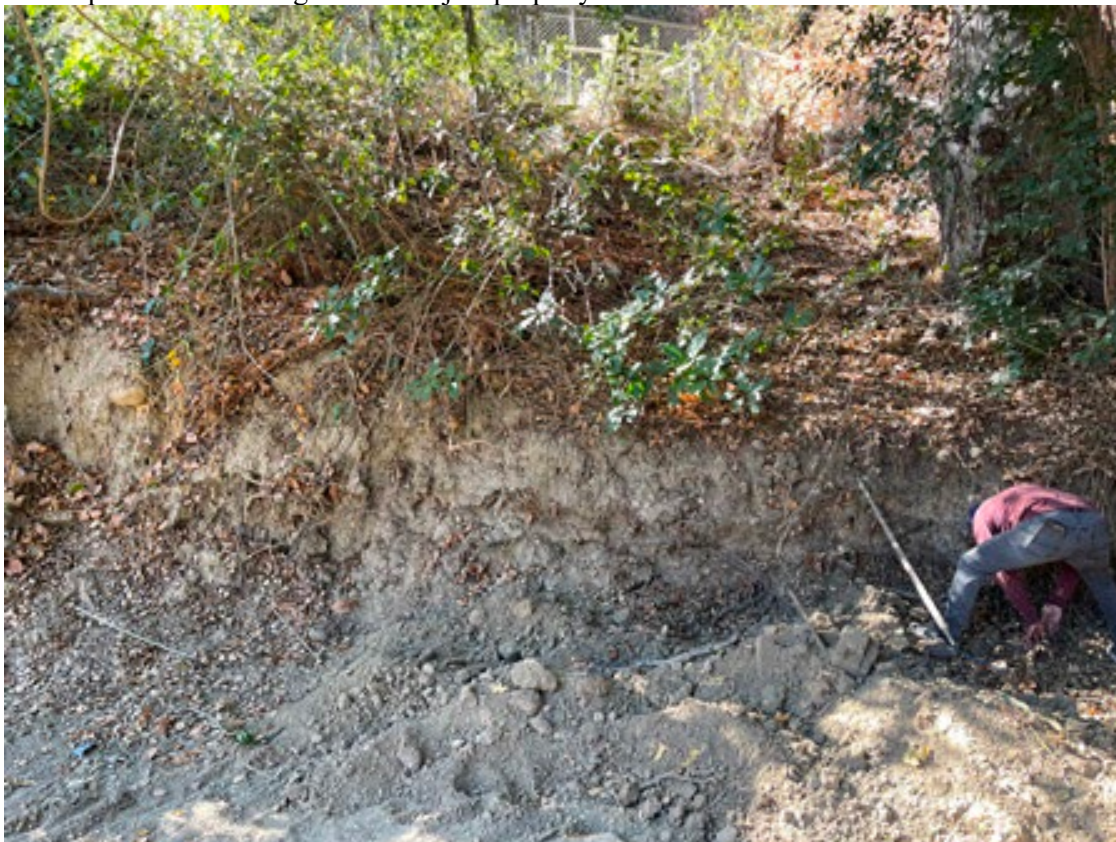
Cut slope at the south edge of the subject property. Oak #3 behind the worker at right.
