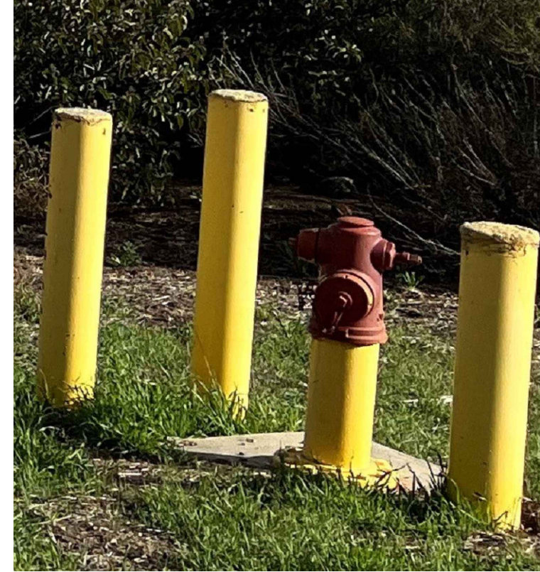
EXISTING FIRE HYDRANT PHOTO (NOT TO SCALE)
